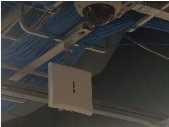
HSM2HOST Located on 1 st floor under CAT5 Tray
